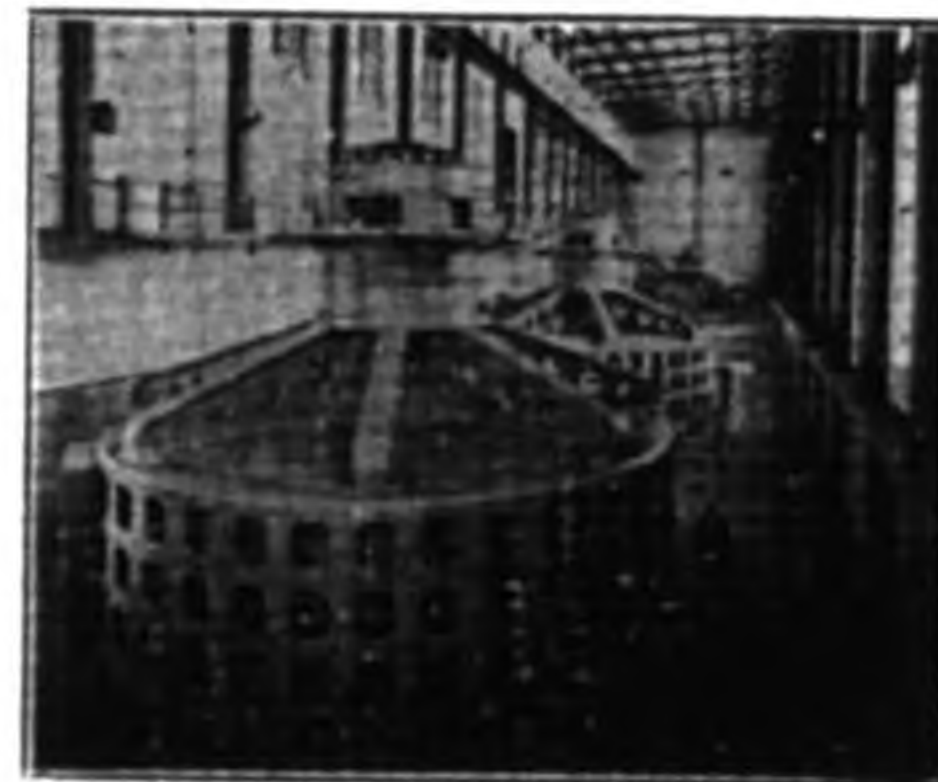
Interior of Chelsea Power House
