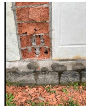
2022 - The Fabrique made no effort to maintain the wall. Meaning, the joints were never resealed and water infiltrated into the back of the bricks.
